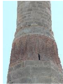
Figure 17. The Bricks Transformative Part of the Minaret, Cut Minaret Mosque after Restoration (Source: Author)
