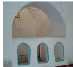
Figure 17: Entrance of the mausoleum from the sanctuary (section A) from the west.
