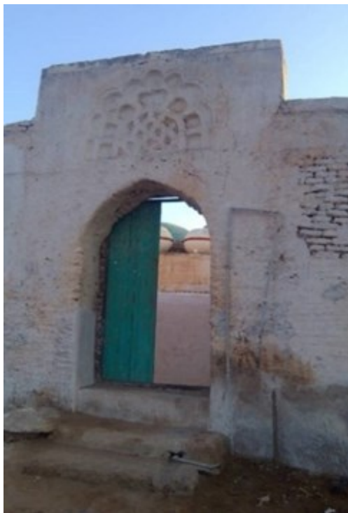
Figure 9: The current main entrance in the northern façade of The Madrasa of Mustafa pasha in Zabid. (Author's photo 2014).
