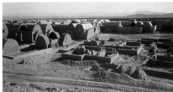
Figure 3. Maadher village under construction, the vaults for roofs. The work of Hassan Fathy has influenced this architecture
