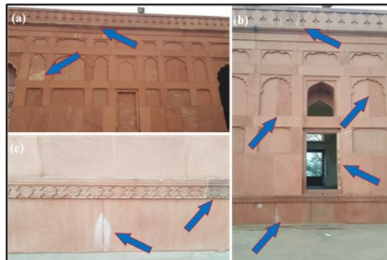
Figure 16. (a, b, c) All these images clearly show the installation of wrong replacements at Badshahi mosque. Source: captured by the author.
