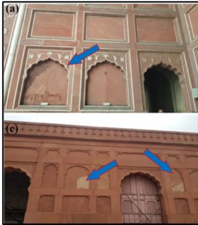
Figure 18. (a, b) Pointing out the incorrect installation of elements at the facade design of Badshahi mosque. Source: captured by the author.
