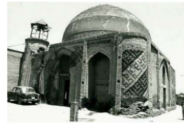
Figure 16. Dome chamber of the Sanjida building before conservation interventions. Damages to the building are visible in the photograph, 1975
