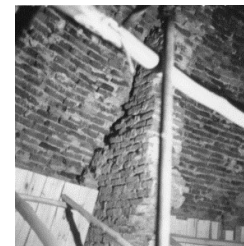
Figure 20. Stiffeners on the inner shell of the dome, 1984 [Documentation Center of Tehran Cultural Heritage Organization]
