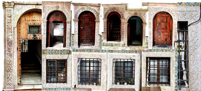
Figure 8. The marble frames of the doors and windows of the Aziza Bey Ottoman palace in Algiers
