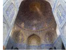
Figure 5. Shah mosque, Isfahan, Iran, Sound bounces back and forth between the floor and ceiling, with the vast dome focusing the sound [53].
