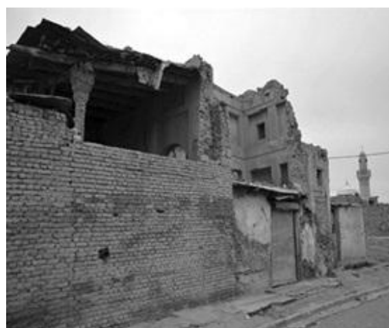
Figure 2: Deterioration of Citadel houses, Erbil (Source: author)
