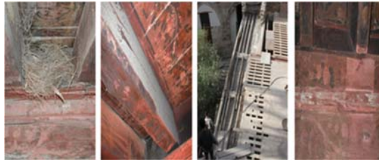
Fig (12 a, b, c, d) The deterioration signs of timber in Al-Razaz house
