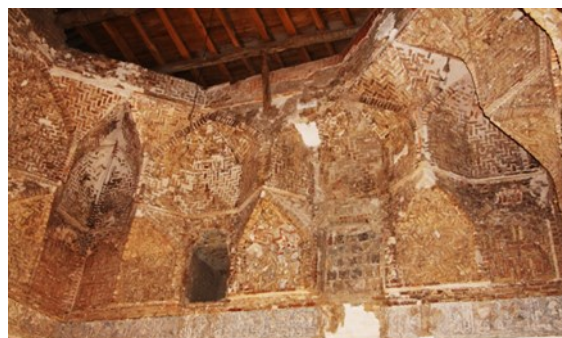
Figure 7. Marand Mosque is an interconnected set of concave units in the transition zone.
