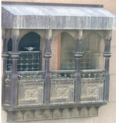
Figure 4: Rowshan in a state of neglect and disuse on the façade of one of the hotels in the Central District, as a result of using the wrong material in constructing Rowshan.
