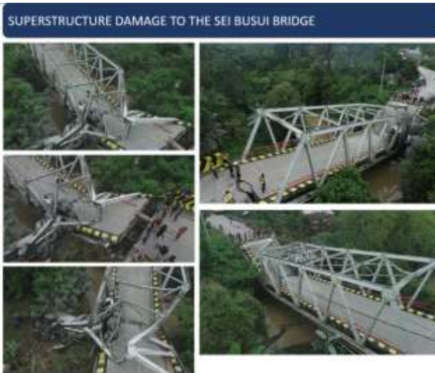
Figure 6. Superstructure damage to the sei busui bridge
