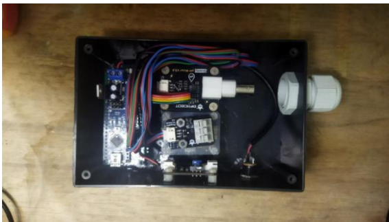
Fig 14 Placement of the entire series of modules and cabling on the project box
