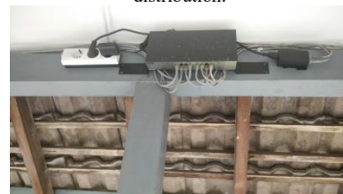
Figure 6. Ceiling-mounted switch for signal extension to isolated areas.
