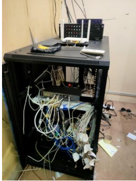
Figure 8. Front view of the server cabinet with powered access point on top.
