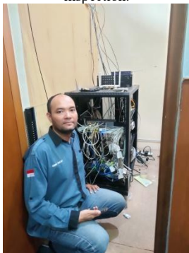
Figure 10. The Main Author beside the server rack showing the scale of cabling setup.
