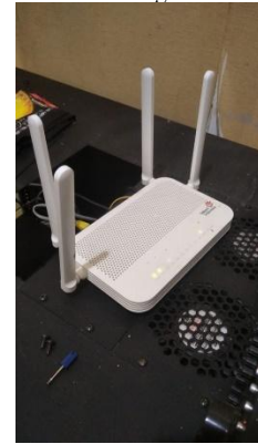
Figure 4. Wireless access point device with multi-antenna configuration.
