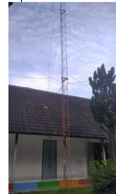
Figure 5. Outdoor antenna tower used for wide area wireless signal distribution.
