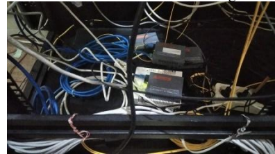
Figure 3. Rear view of the network cabinet showing cable distribution and switch configuration.
