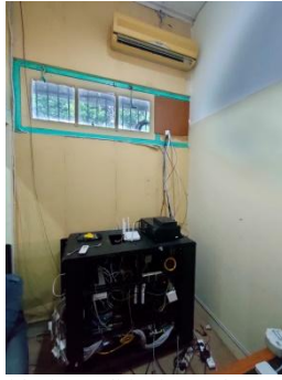
Figure 7. Server room with air conditioning and external cable entry points.
